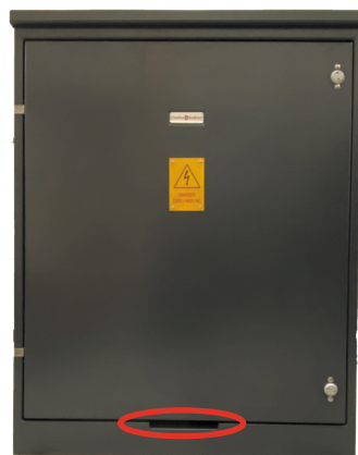
Cable exit tray
