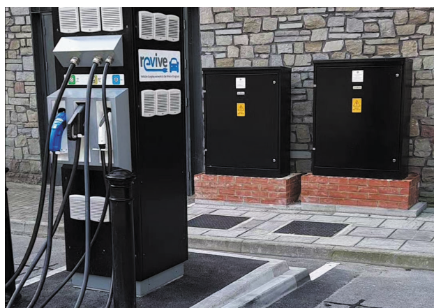
Bespoke, slimline pillar supplying EV Chargers.
