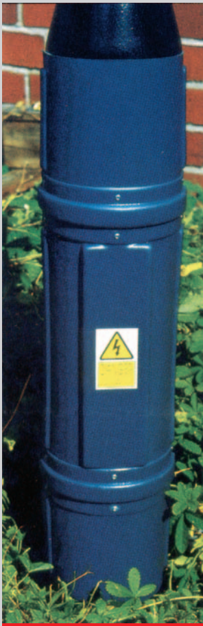
SD EMERGENCY DOOR
