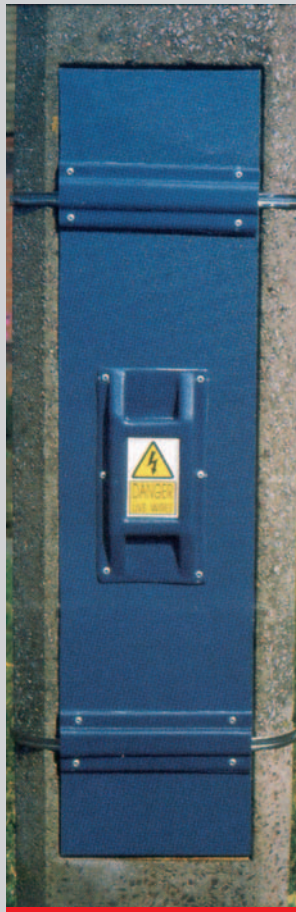
FSD EMERGENCY DOOR
